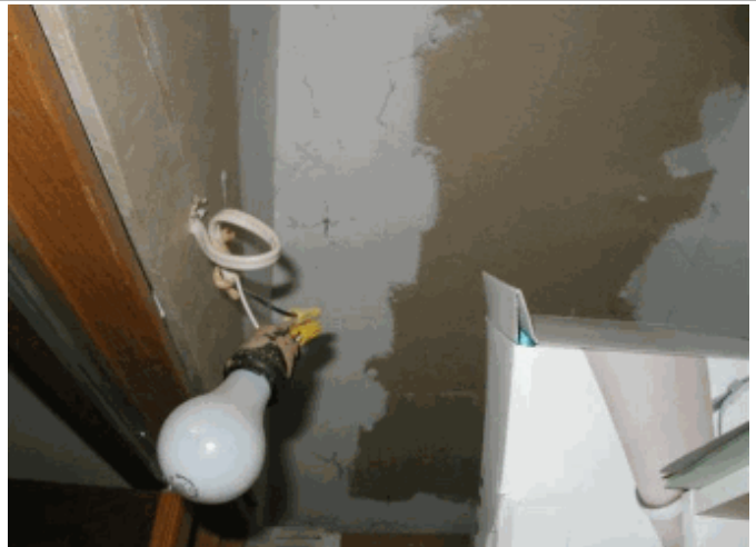
Bedroom closet has unsafe light, is a fire hazard, install pertinent fluorescent light
