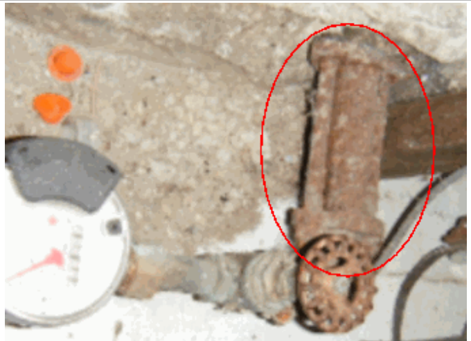
Old iron pipe water entry into the house, could need replacement at any time
