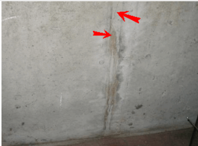
Crack in foundation wall is NOT a structural concern, some water weeps in
