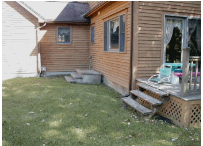
Remove concrete steps and correct yard drainage to shed water away
