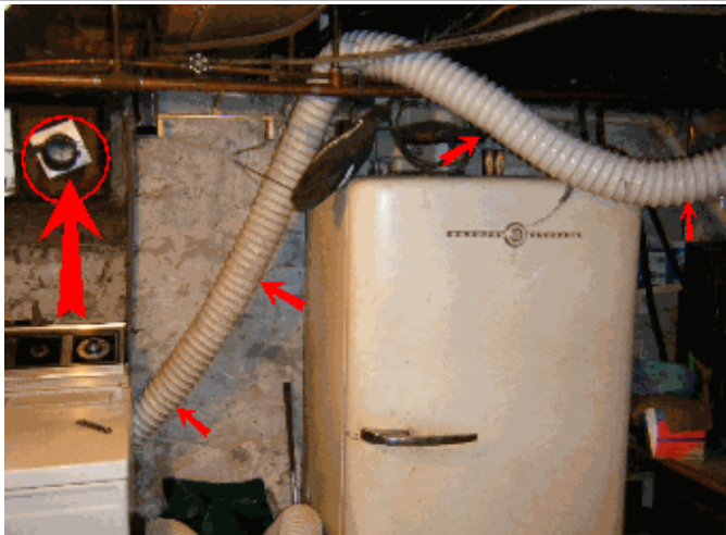
Replace dryer vent with a metal pipe and vent to the outside
