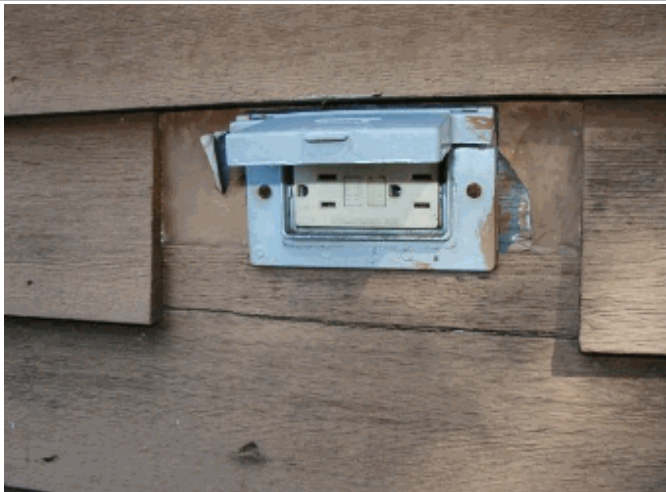
GFCI receptacle above deck does not trip off, and wood trim missing around cover
