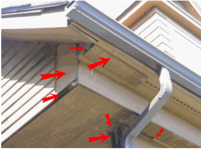
Exterior: Missing molding outside
