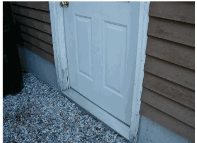
Exterior: Paint trim on garage door to avoid wood rot
