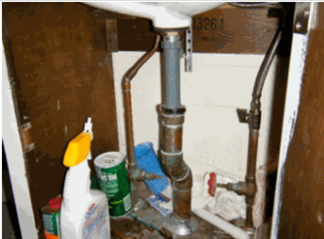
No apparent trap; have plumber evaluate and correct as needed.
