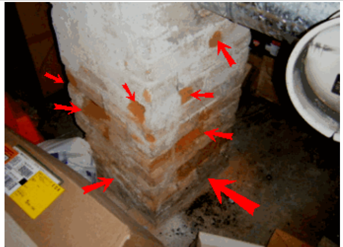
Bricks at bottom of original chimney are deteriorated; rebuild
