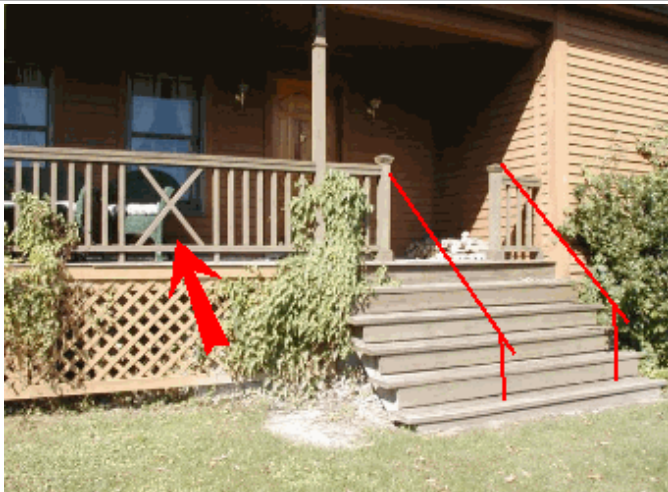
Add handrails along steps and openings below handrail too large in areas
