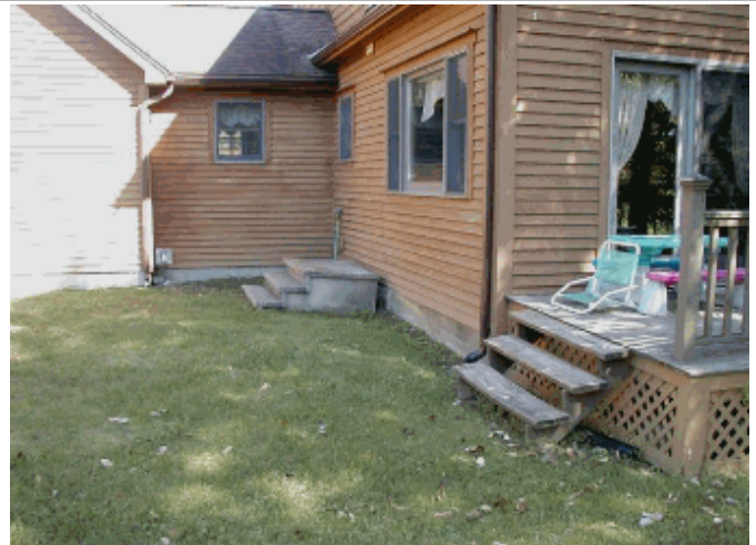
Remove concrete steps and correct yard drainage to shed water away
