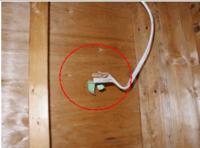
Elect.: Terminate free end wires in boxes, this one in garage one under window in bedr
