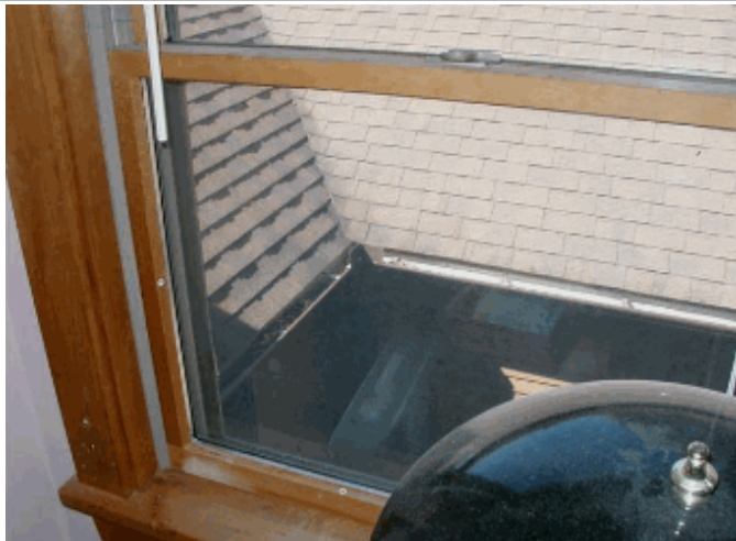
Glass is fogged, replace glass to make clear
