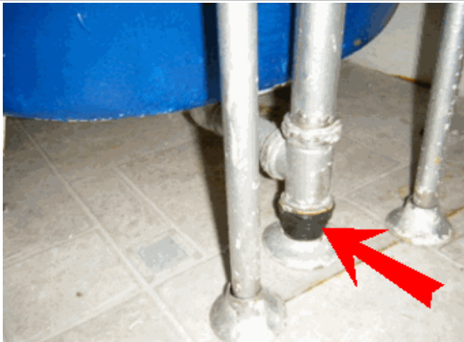
Tape on drain pipe at floor; correct, may need to cut open the floor
