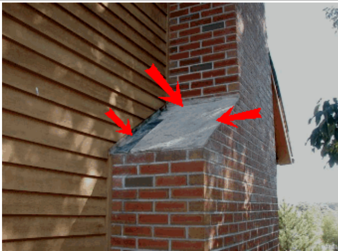
Exterior: Flag stone missing from chimney
