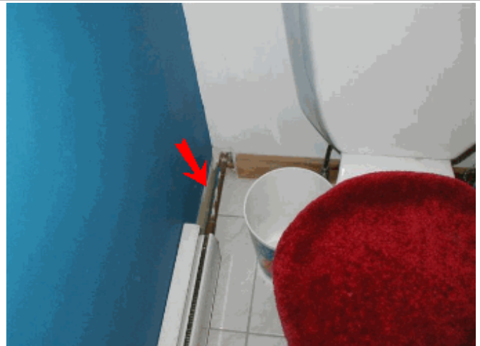
Trim missing in many areas and radiator cover missing too
