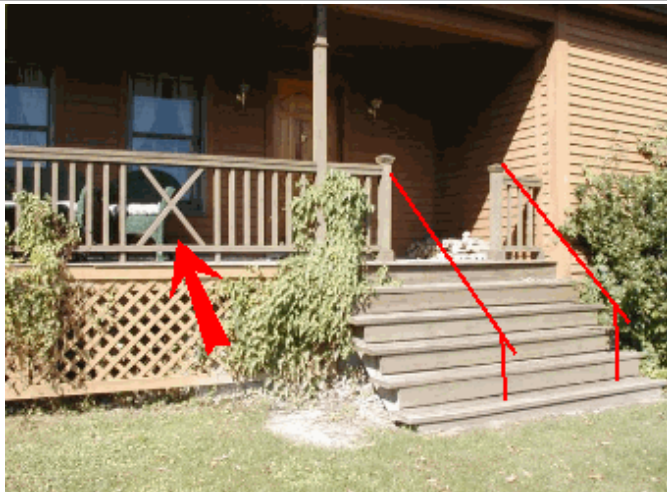
Add handrails along steps and openings below handrail too large in areas
